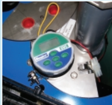
Controller Capable Of Nine Flushes Per Day! Operates With 9 Volt Battery
